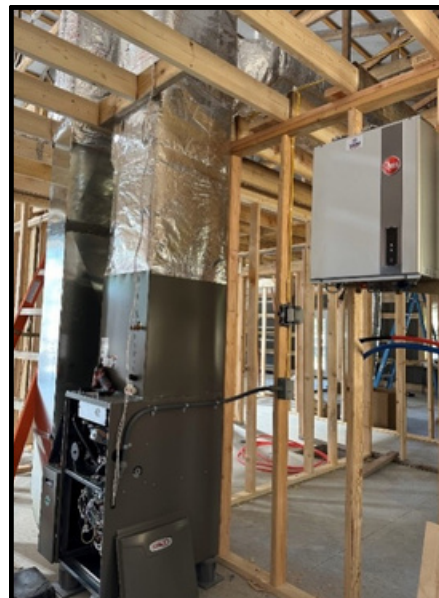
Lennox HVAC and Rheem water heater installation.
